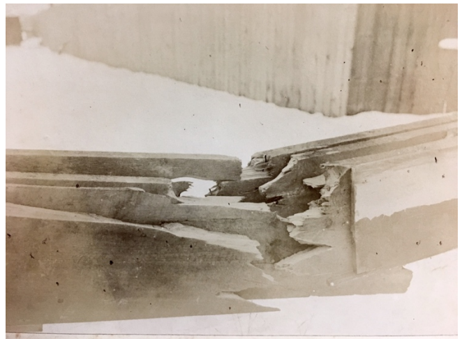
The beam that supported the second floor
